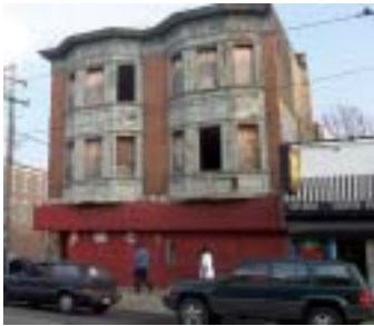
Vacancy and dilapidated structures are a significant issue on Chester Avenue.
